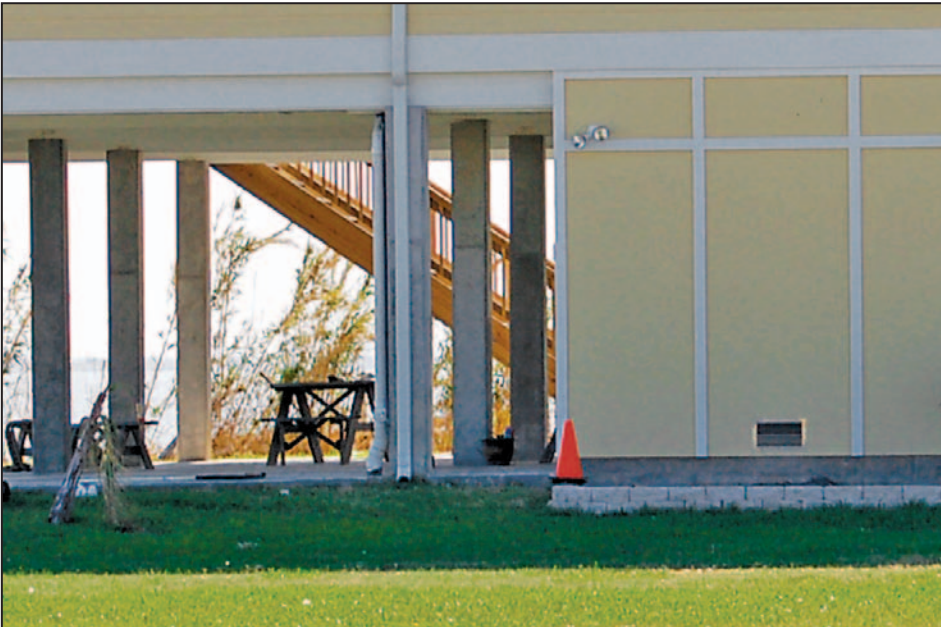
Figure 2-20. Flood opening in an enclosure with breakaway walls, Hurricane Ike (Galveston Bay shoreline, San Leon, TX)
