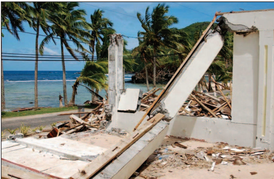
Figure 3-12. Damage from the 2009 tsunami (Amanave, American Samoa)
