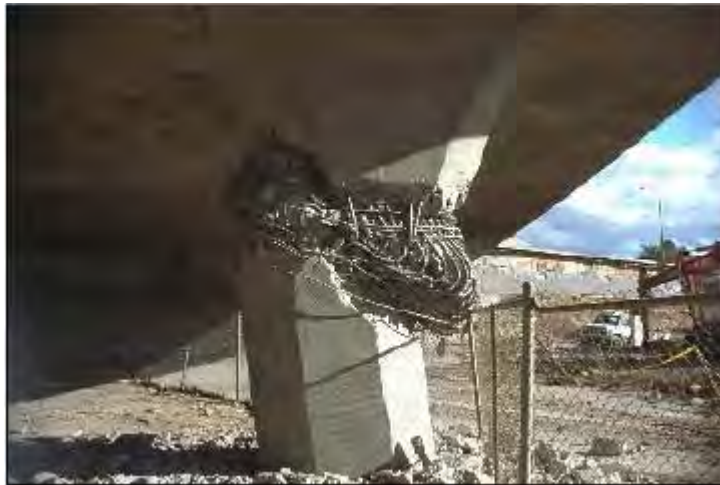
Figure D-15 Earthquake Damage (Source: FEMA)
